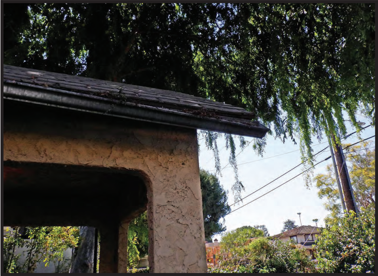
Damaged Eave on West Elevation of Residence at 1022 La Cadena Avenue, Arcadia, CA (SSW)
