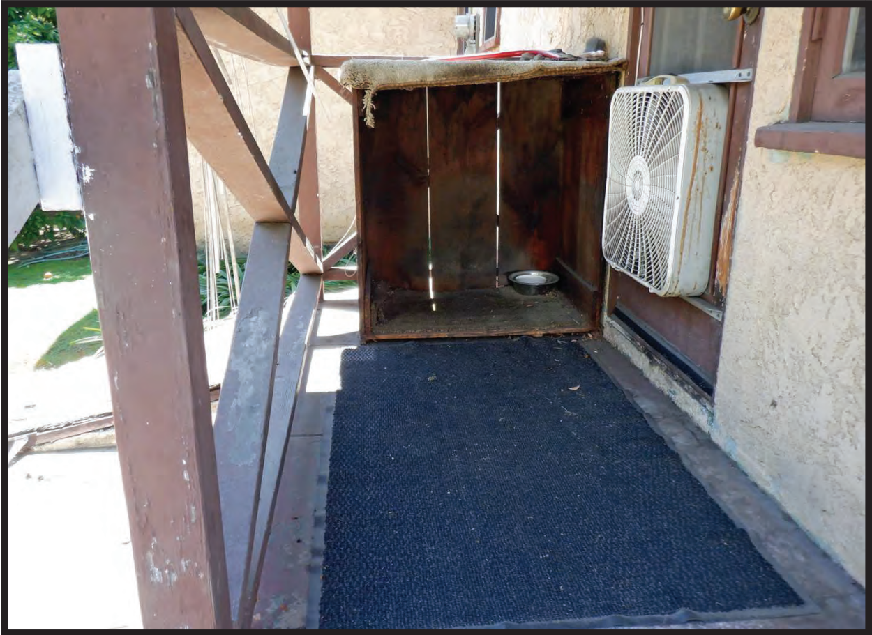
Rear Porch, East Elevation of Residence at 1022 La Cadena Avenue, Arcadia, CA (W)
