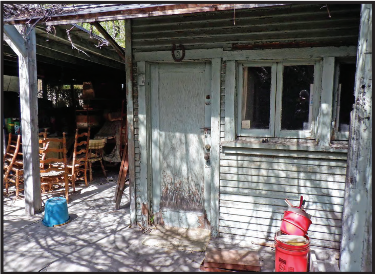
South Elevation of Western End of Large Barn/Workshop, 1022 La Cadena Avenue, Arcadia, CA (NNW)
