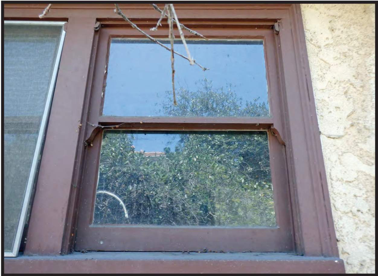
Window Detail, North Elevation of Residence at 1022 La Cadena Avenue, Arcadia, CA (S)
