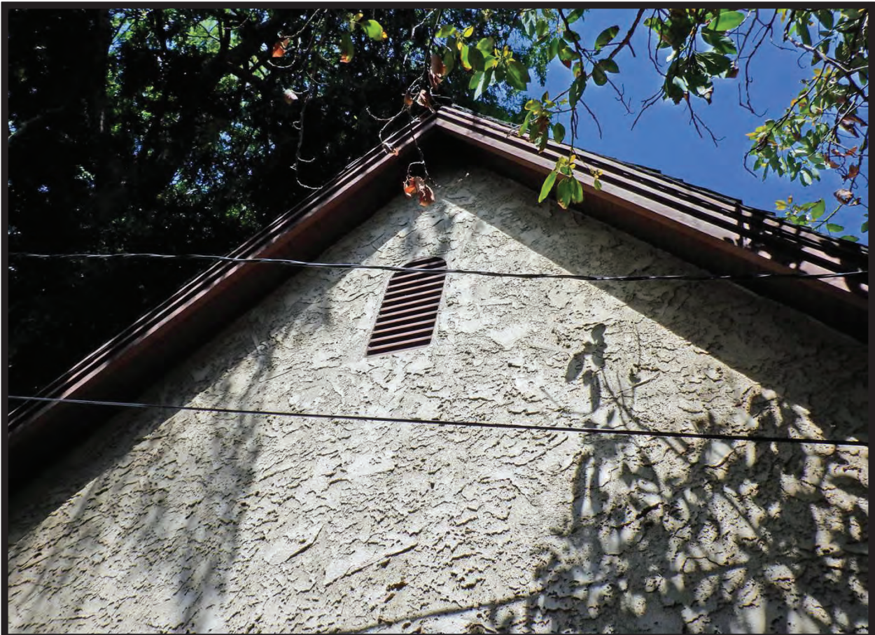
Roof Peak, South Elevation of Residence at 1022 La Cadena Avenue, Arcadia, CA (N)
