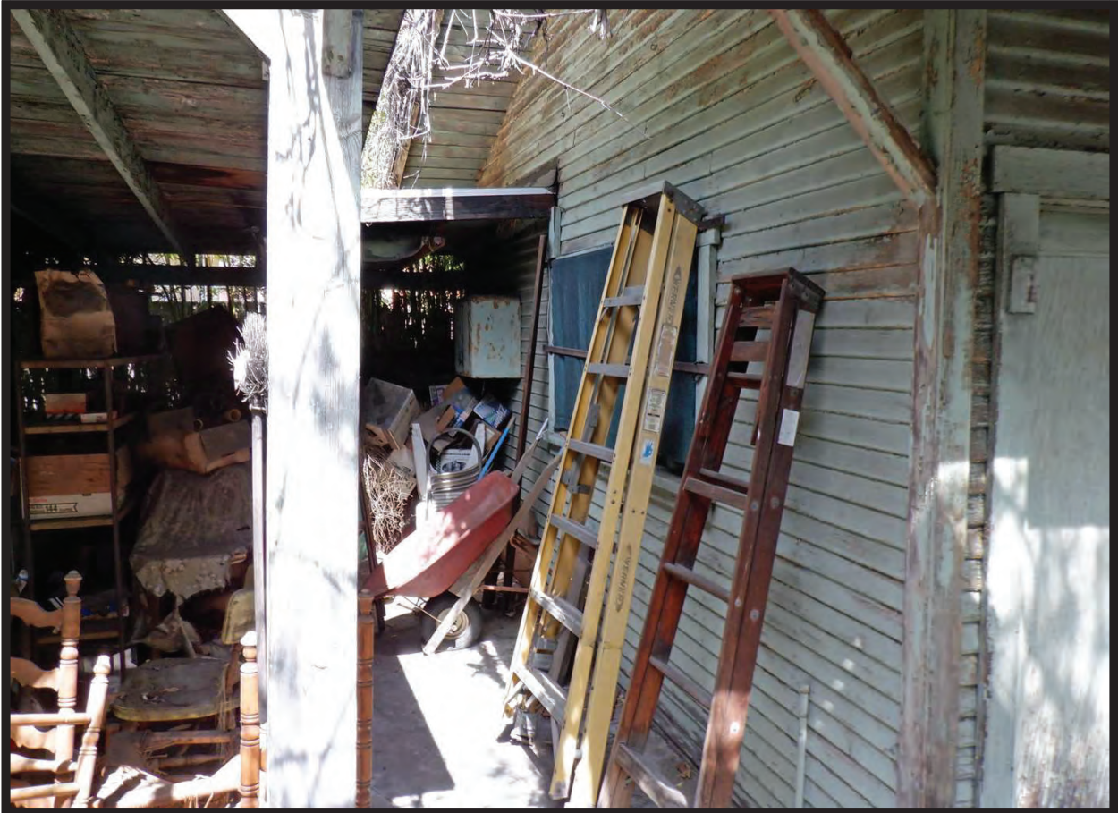
West Elevation of Western Eil of Large Barn/Workshop, 1022 La Cadena Avenue, Arcadia, CA (NNE)
