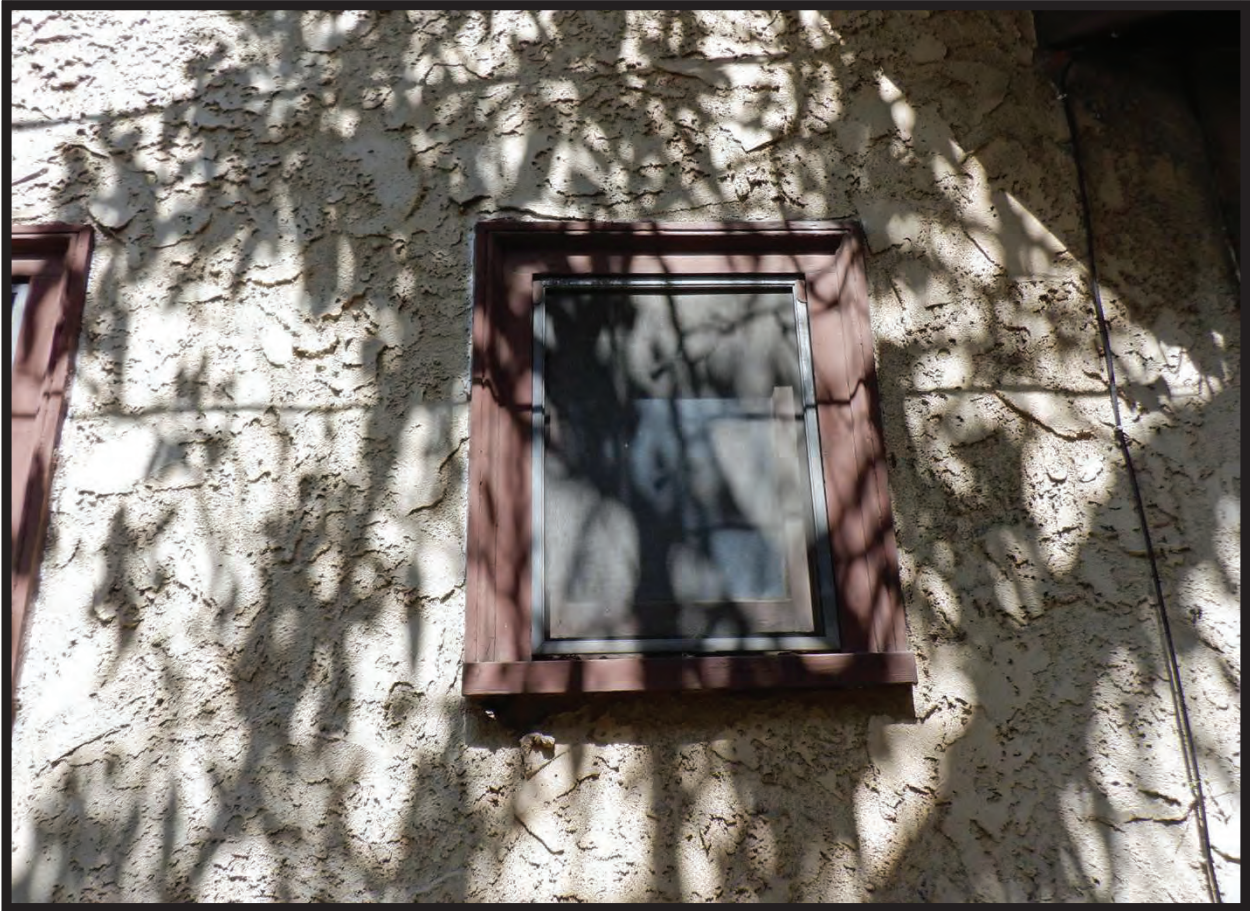
Window Detail, South Elevation of Residence at 1022 La Cadena Avenue, Arcadia, CA (N)
