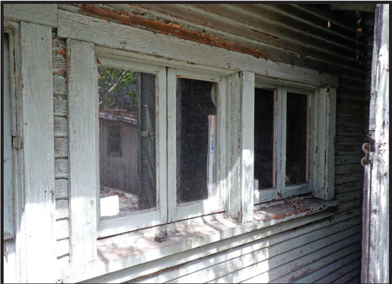
Window Detail, South Elevation of Western Ell of Large Barn/Workshop, 1022 La Cadena Avenue, Arcadia, CA (ENE)
