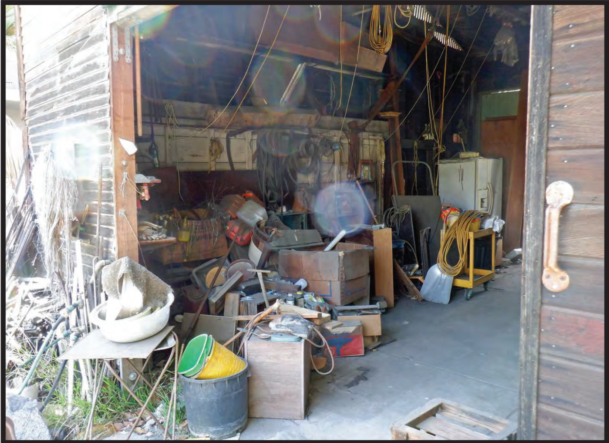
Detail, East Elevation of Large Barn/Workshop with Bay Door, 1022 La Cadena Avenue, Arcadia, CA (WSW)
