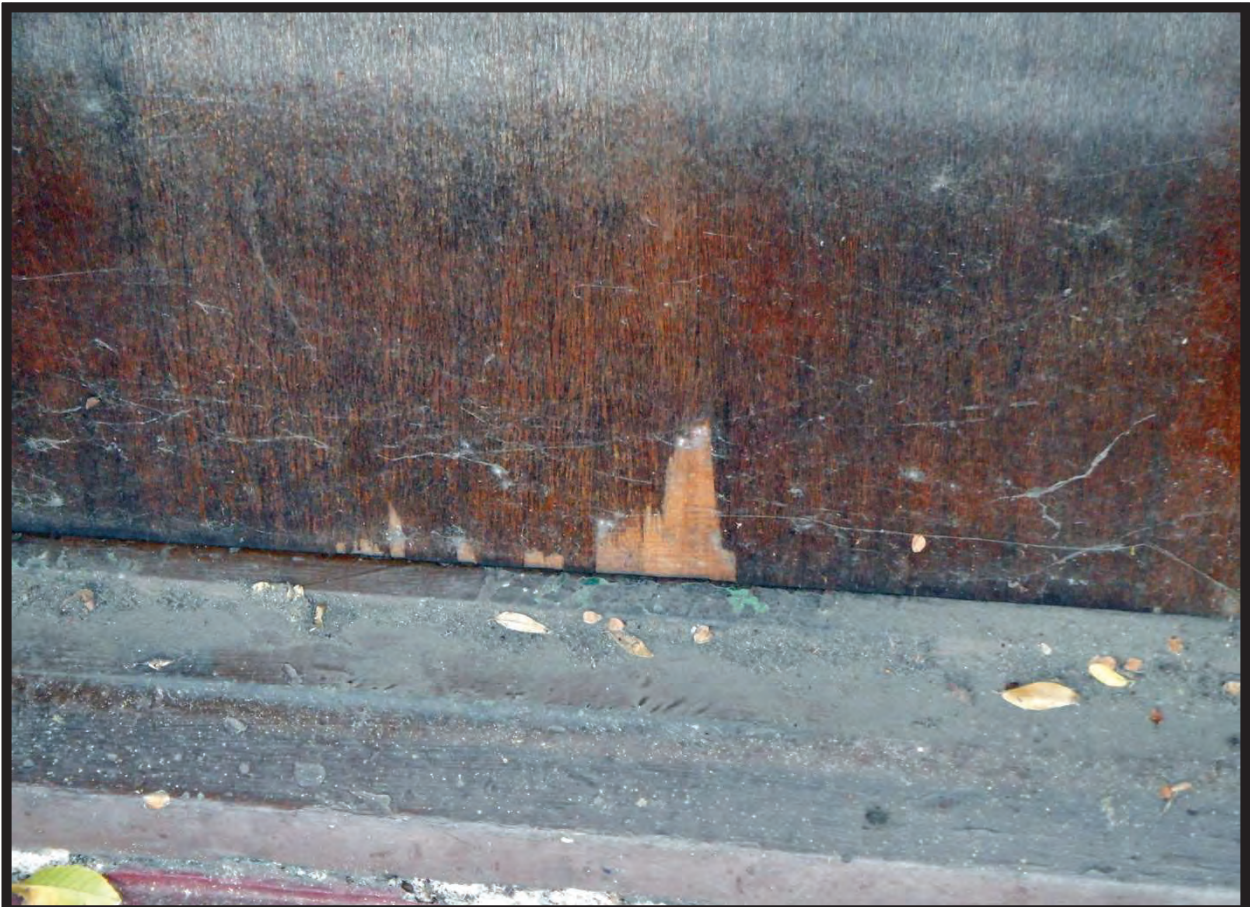
Veneer Damage on Main Entry Door, West Elevation of Residence at 1022 La Cadena Avenue, Arcadia, CA (E)
