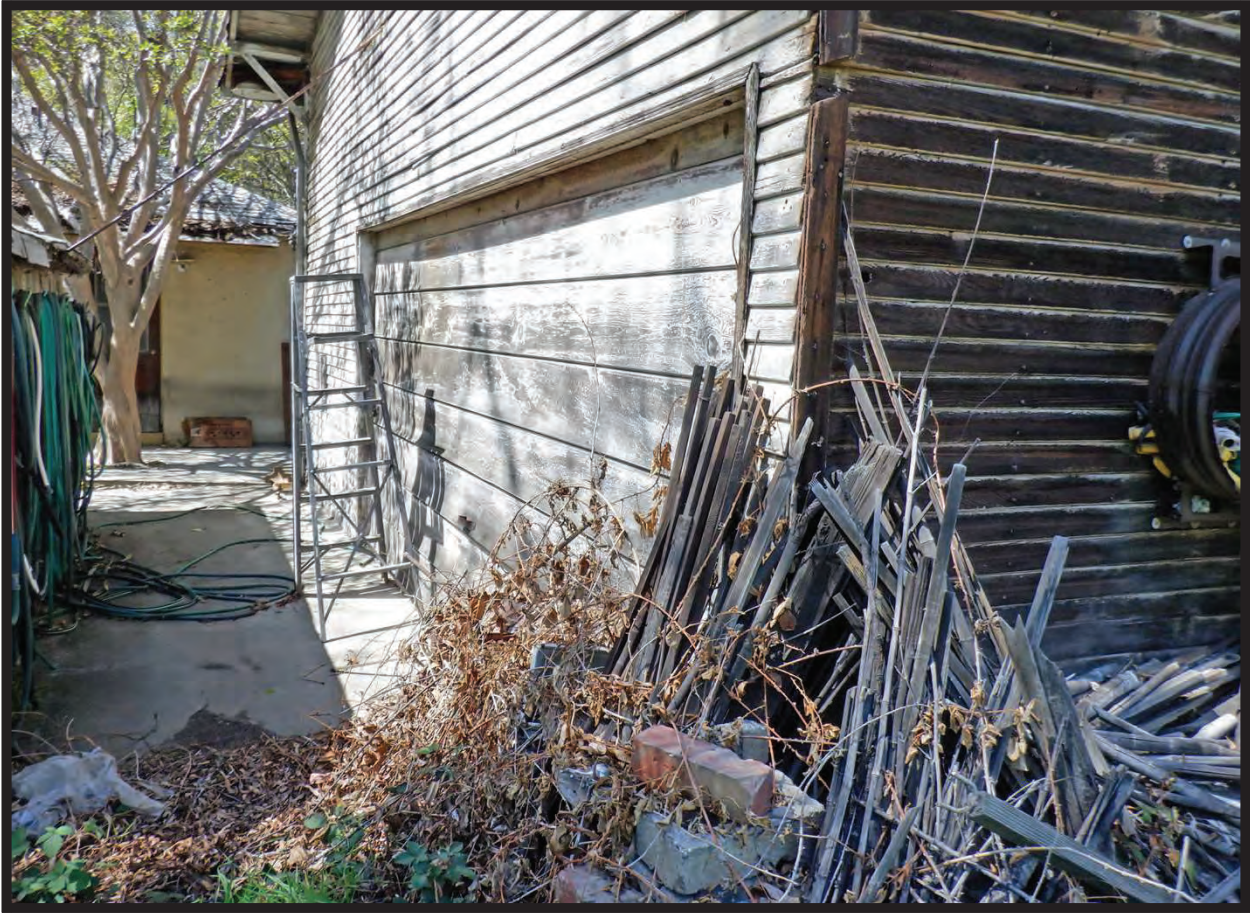
South Elevation of Large Barn/Workshop with Bay Door, 1022 La Cadena Avenue, Arcadia, CA (WNW)
