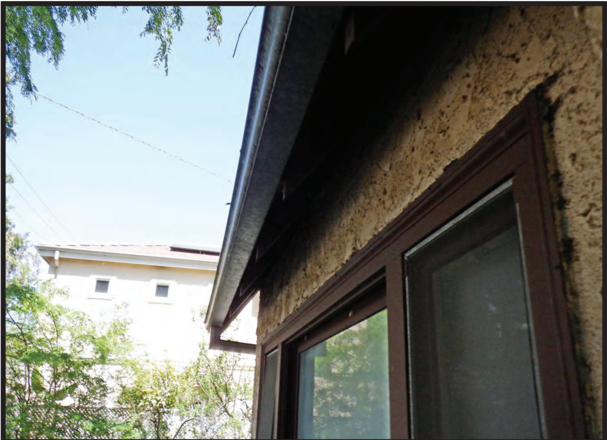
Eave Detail, West Elevation of Residence at 1022 La Cadena Avenue, Arcadia, CA (NNE)
