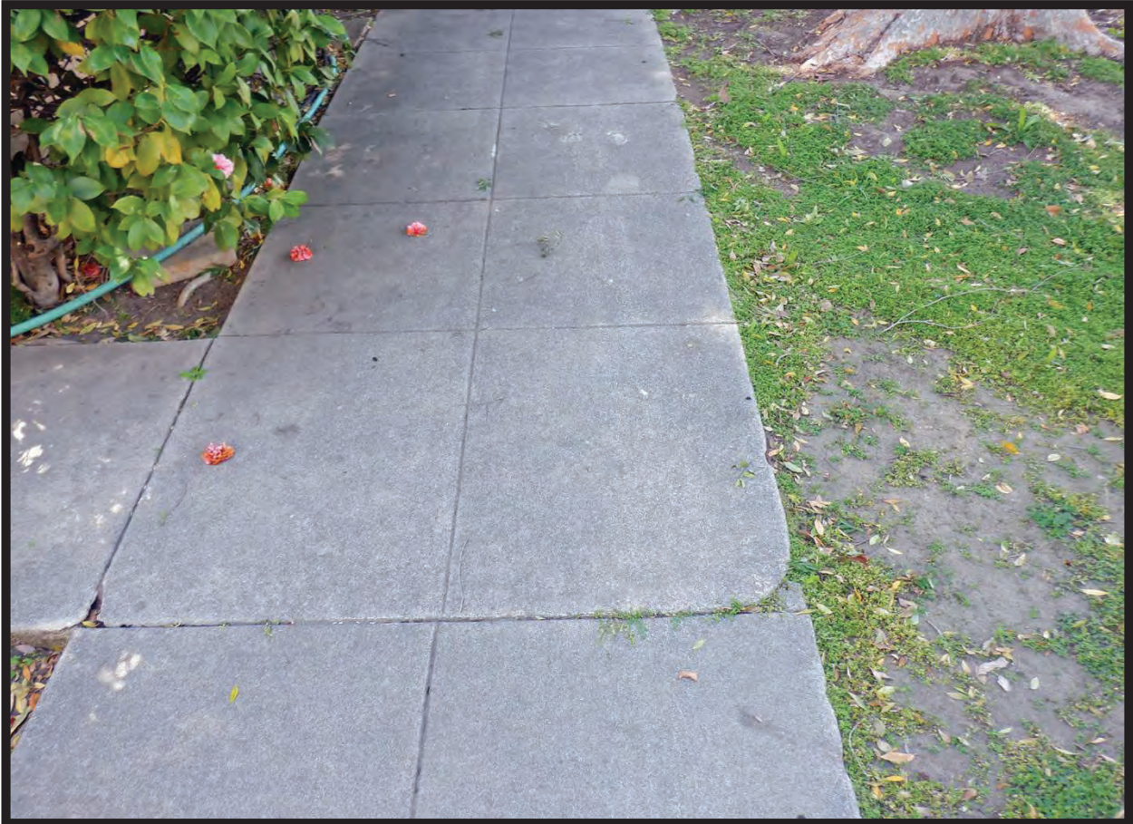
Concrete Walkway on West Elevation of Residence at 1022 La Cadena Avenue, Arcadia, CA (S)
