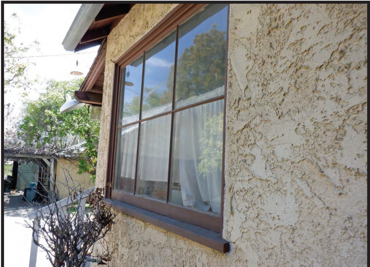
Window Detail, North Elevation of Residence at 1022 La Cadena Avenue, Arcadia, CA (ESE)
