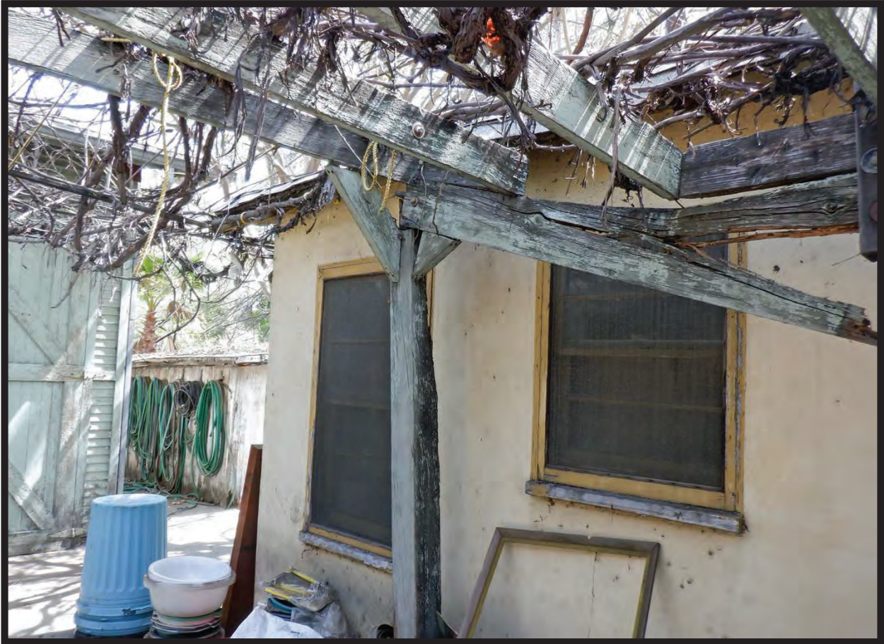
Falling Roof on North Elevation of 1944 Residence, 1022 La Cadena Avenue, Arcadia, CA (SE)
