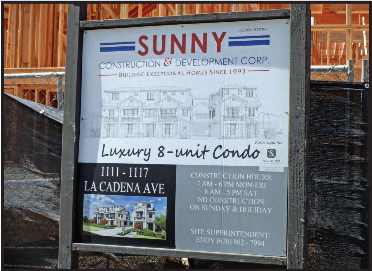
Signage at Construction Site, Arcadia, CA.
