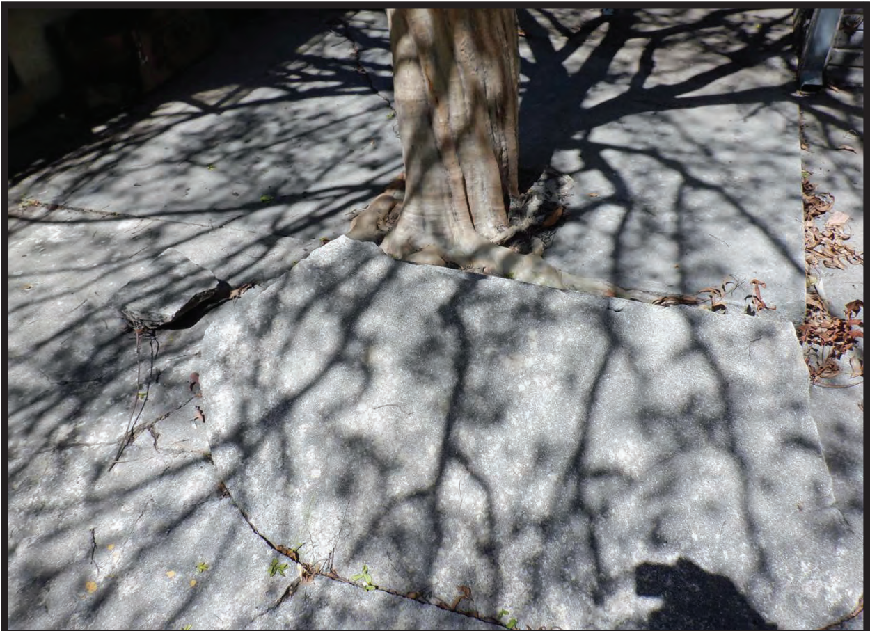
Broken Concrete Pad West of Shed at 1022 La Cadena Avenue, Arcadia, CA (N)
