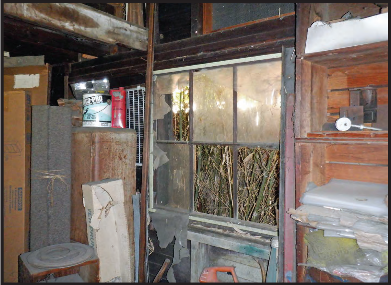
Interior Detail, Large Barn/Workshop with Bay Door, 1022 La Cadena Avenue, Arcadia, CA (NNW)
