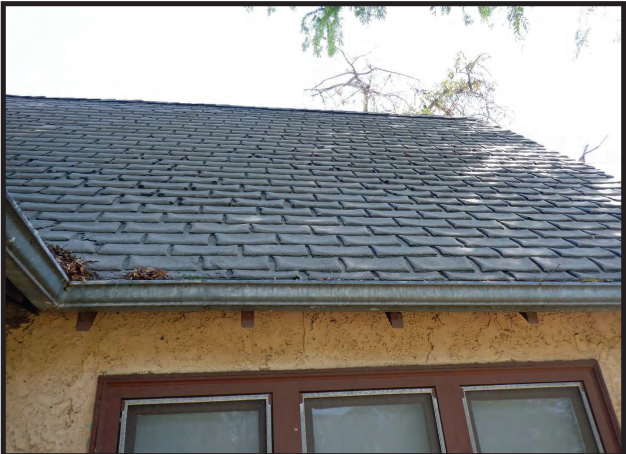
Roof Detail, West Elevation of Residence at 1022 La Cadena Avenue, Arcadia, CA (ESE)
