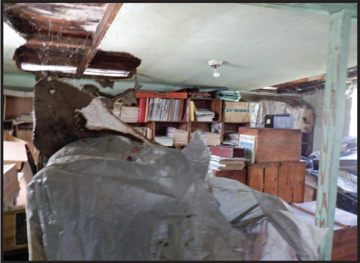
Interior of Shed East of 1944 Residence at 1022 La Cadena Avenue, Arcadia, CA (N)
