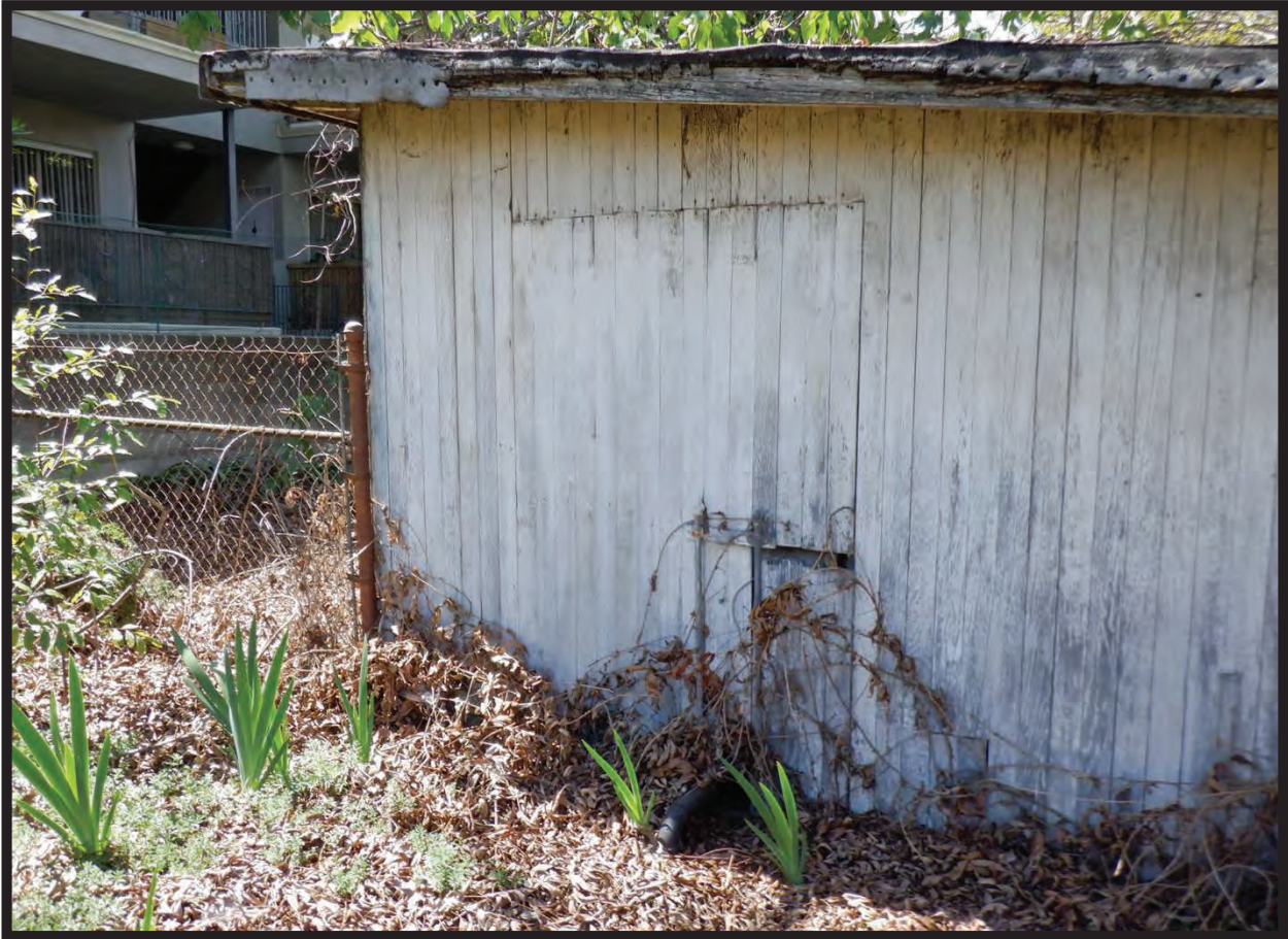
East Elevation of Shed East of 1944 Residence at 1022 La Cadena Avenue, Arcadia, CA (WSW)
