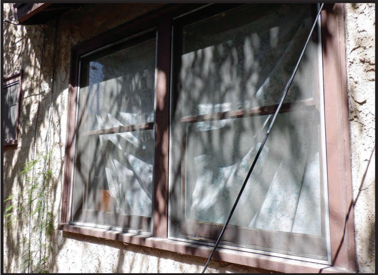
Window Detail, South Elevation of Residence at 1022 La Cadena Avenue, Arcadia, CA (NW)
