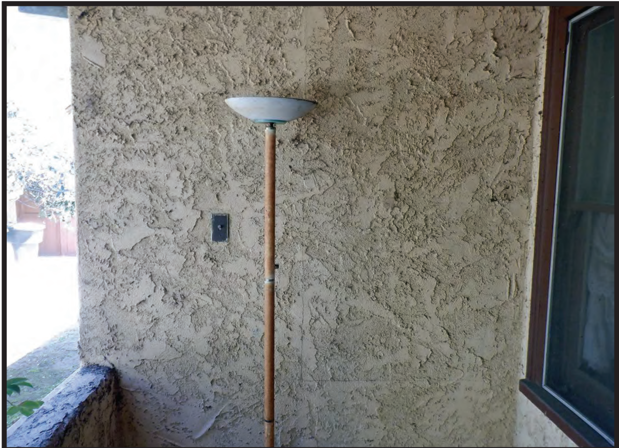
Wall Detail, Side Porch, North Elevation of Residence at 1022 La Cadena Avenue, Arcadia, CA (E)
