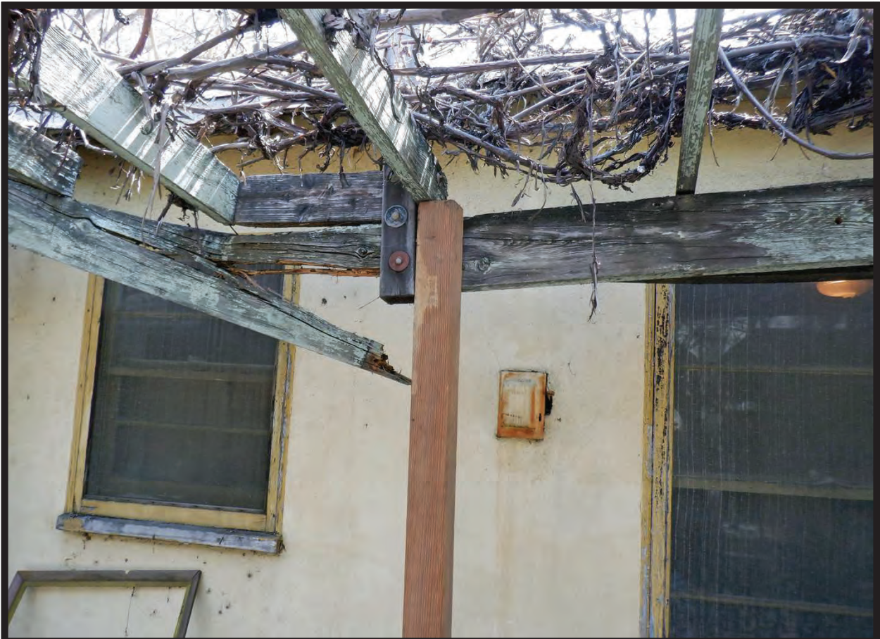
Falling Roof on North Elevation of 1944 Residence, 1022 La Cadena Avenue, Arcadia, CA (S)
