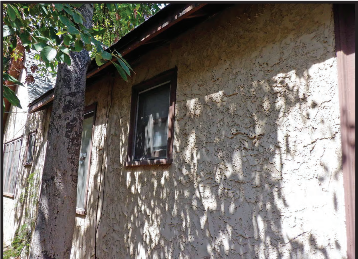
Window Detail, South Elevation of Residence at 1022 La Cadena Avenue, Arcadia, CA (NW)
