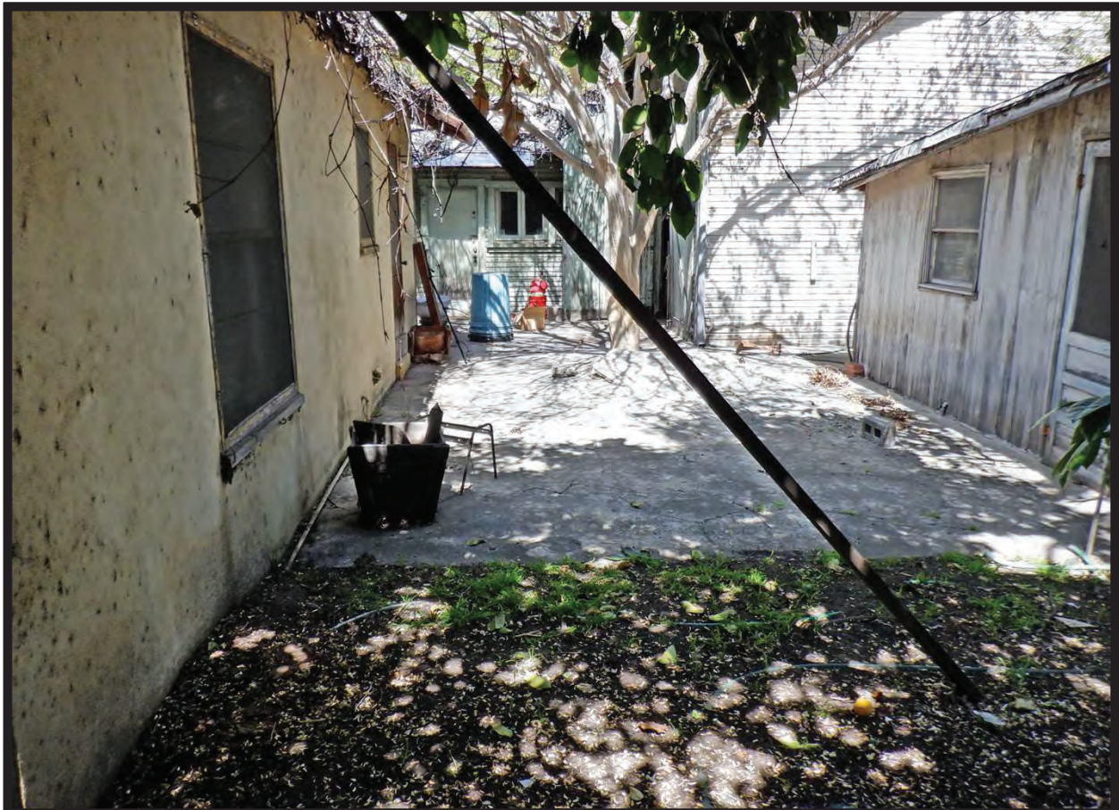
East Elevation of 1944 Residence and West Elevation of Shed at 1022 La Cadena Avenue, Arcadia, CA (N)
