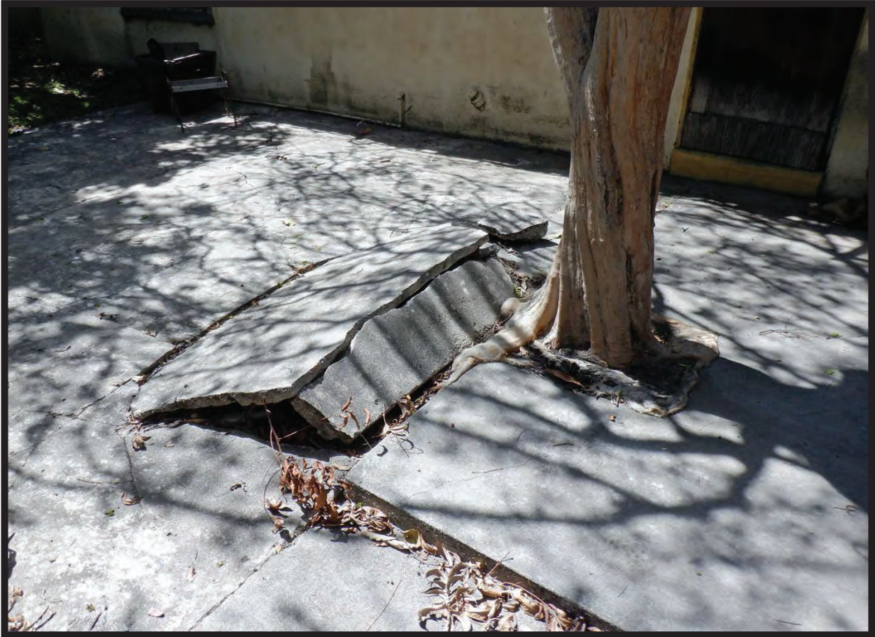
Broken Concrete Pad West of Shed at 1022 La Cadena Avenue, Arcadia, CA (WSW)
