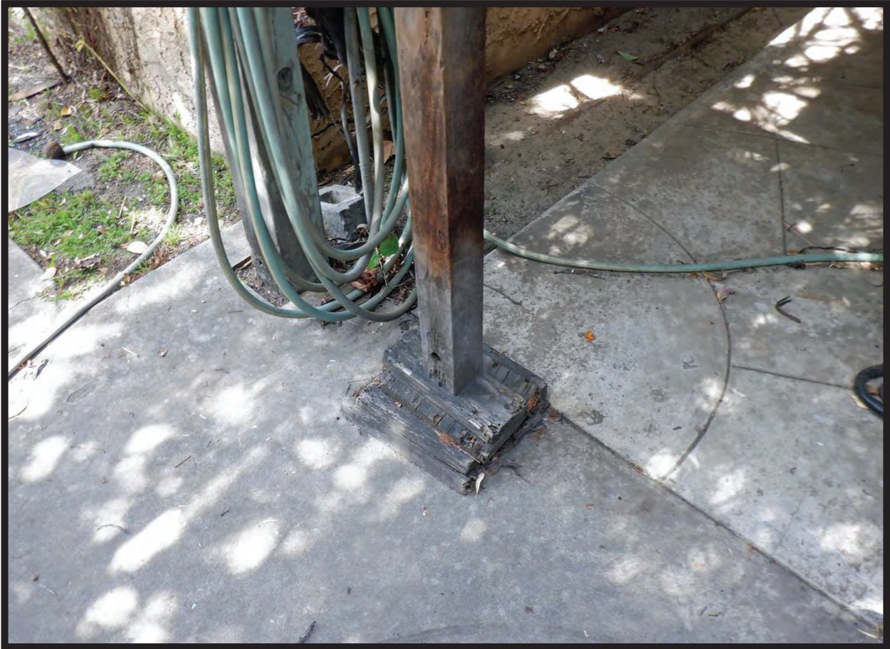
Detail on Covered Patio between Office and Garage, 1022 La Cadena Avenue, Arcadia, CA (NW)
