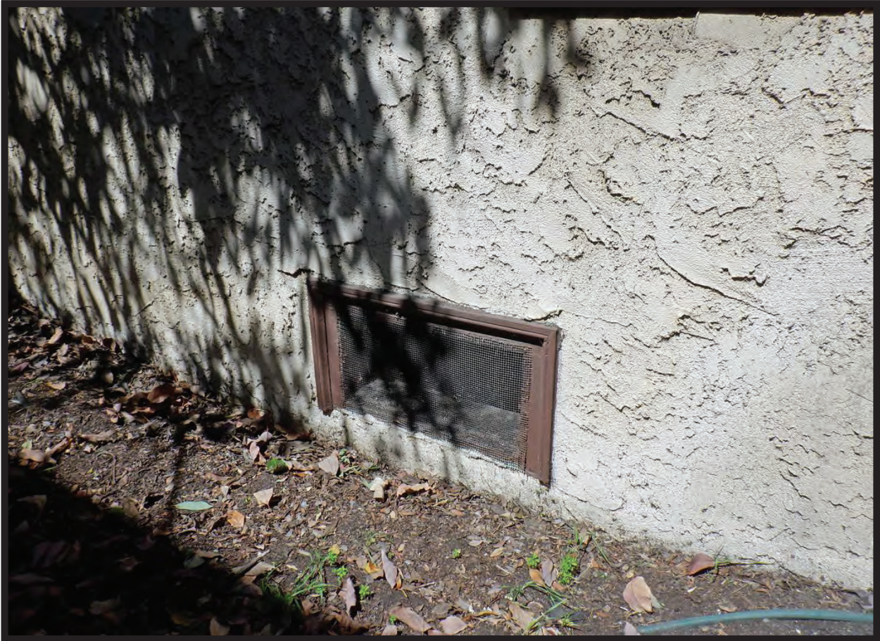
Crawl Space Entry, South Elevation of Residence at 1022 La Cadena Avenue, Arcadia, CA (NW)
