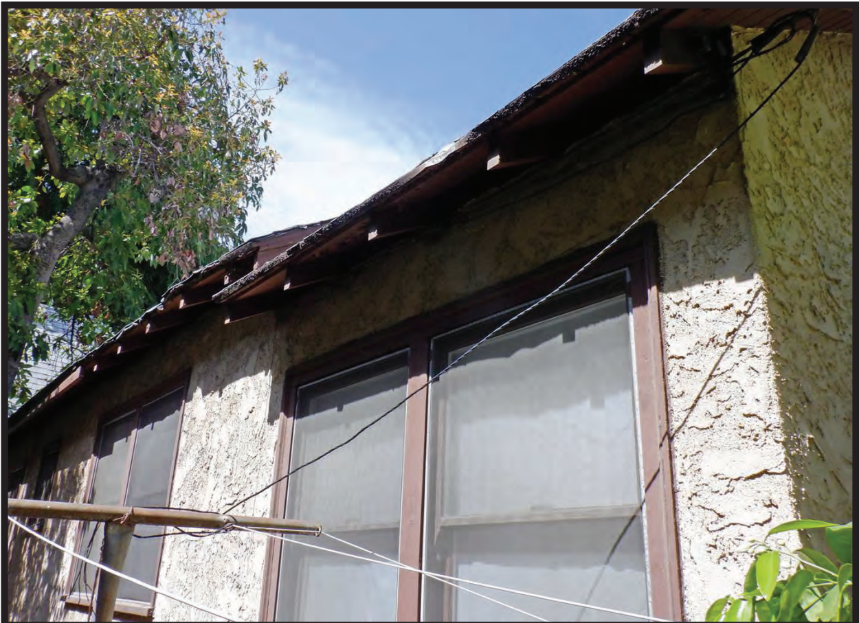
Roof Lines on South Elevation of Residence at 1022 La Cadena Avenue, Arcadia, CA (NW)
